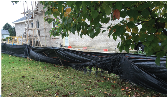
IMPROPER SILT FENCE INSTALLATION
